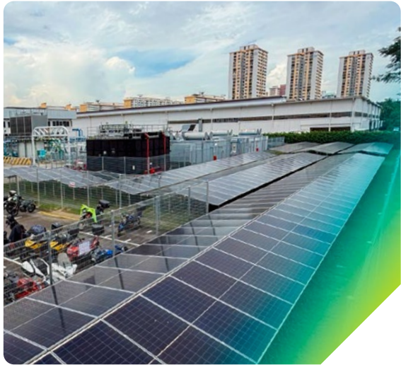
Newly installed solar PV system at NCS Bedok
